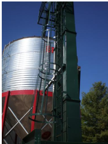
Silo and Bucket Elevator
