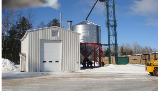
From left to right: Boiler building, Pellet silo, Dumping Station
