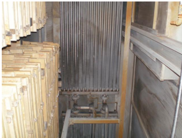
Coils and heat pipes within Kiln
