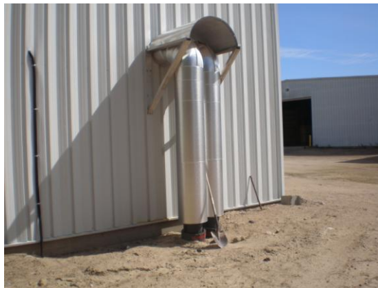
Pipes leaving Boiler room going underground to service buildings
