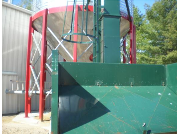
Silo and Bucket Elevator and Dumping Station
